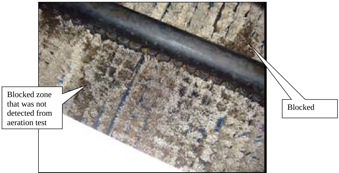
Figure 7.2.3.5 Clear and blocked bundles
