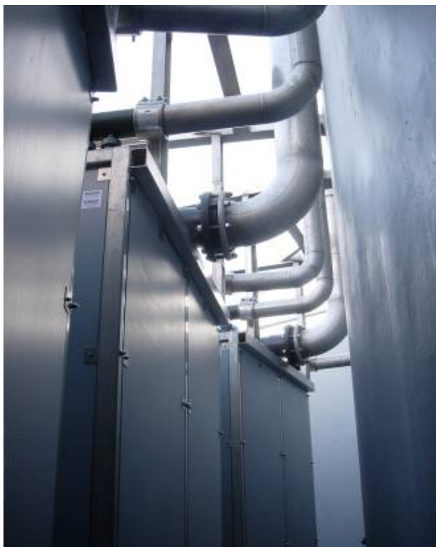
Figure 6.3.12.2: Permeate Header Connection.
