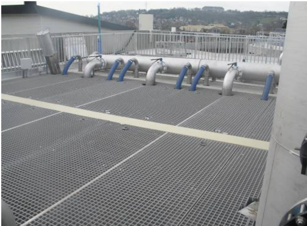
Figure 7.2.3.3 Aeration pattern – masked by grating
